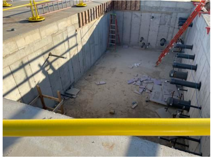
Lower level of Equipment/Pump House Taken on Sep 1, 2023, 7:41 AM CDT Added on Sep 3, 2023, 6:52 AM CDT Added by andrew gordon
