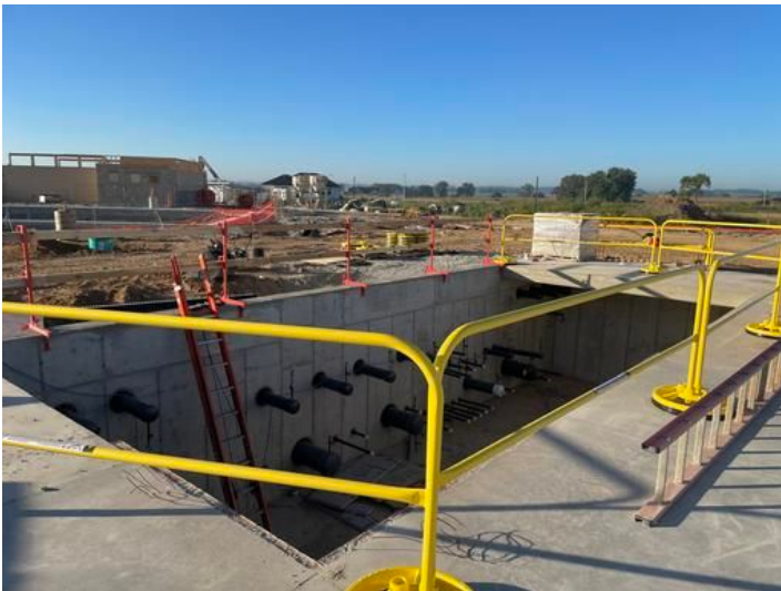
Safety of Equipment/Pump House Taken on Sep 1, 2023, 7:41 AM CDT Added on Sep 3, 2023, 6:51 AM CDT Added by andrew gordon
