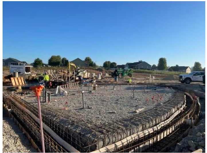
Prepare lazy River entry for Concrete pour. Taken on Sep 1, 2023, 7:38 AM CDT Added on Sep 3, 2023, 6:53 AM CDT Added by andrew gordon
