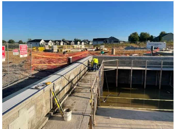
Finishes going on at Lap Pool Taken on Sep 1, 2023, 7:37 AM CDT Added on Sep 3, 2023, 6:53 AM CDT Added by andrew gordon
