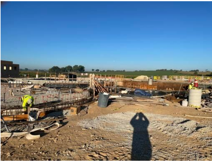
Prepare Lazy River entry for concret pour Taken on Sep 1, 2023, 7:39 AM CDT Added on Sep 3, 2023, 6:52 AM CDT Added by andrew gordon
