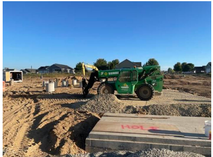
Prepare for concrete pour of Waterside run out pad Taken on Sep 1, 2023, 7:39 AM CDT Added on Sep 3, 2023, 6:52 AM CDT Added by andrew gordon
