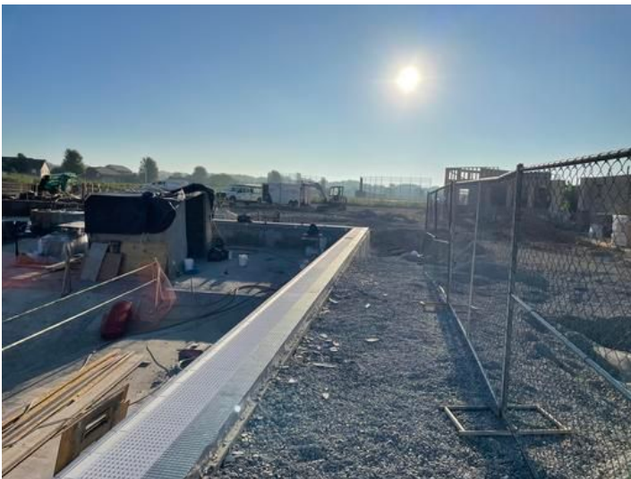
Install finishes on Lap Pool Taken on Sep 1, 2023, 7:37 AM CDT Added on Sep 3, 2023, 6:53 AM CDT Added by andrew gordon
