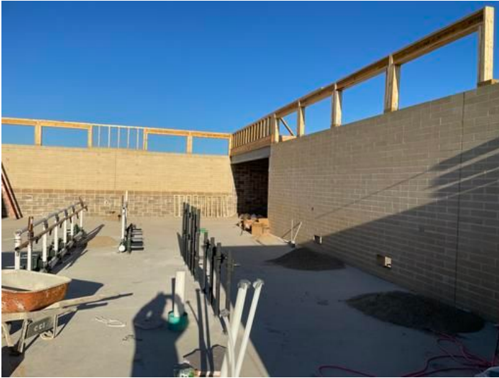
Installation of Plumbing rough in Taken on Sep 1, 2023, 7:55 AM CDT Added on Sep 3, 2023, 6:52 AM CDT Added by andrew gordon
